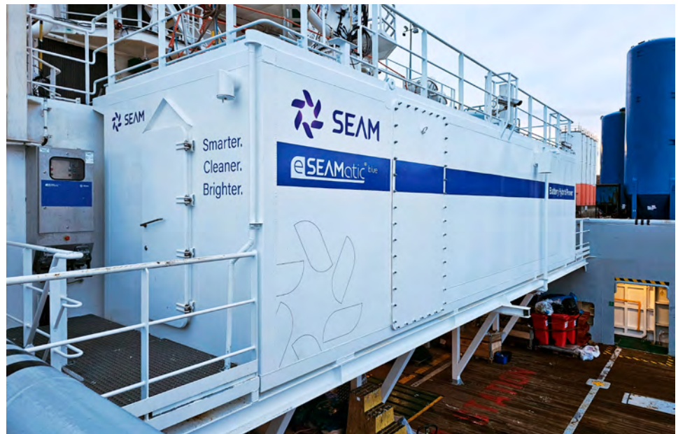
Frost Tide hybrid battery installation.
